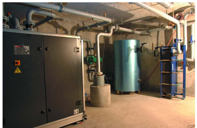
Ground-water heat pump, well and exchanger in a mechanical room
