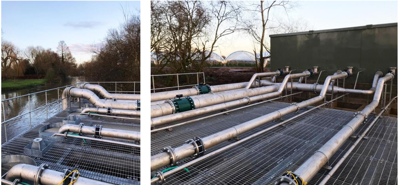
Pipes extract water from the river and supply it to the nearby heat pump plant room
