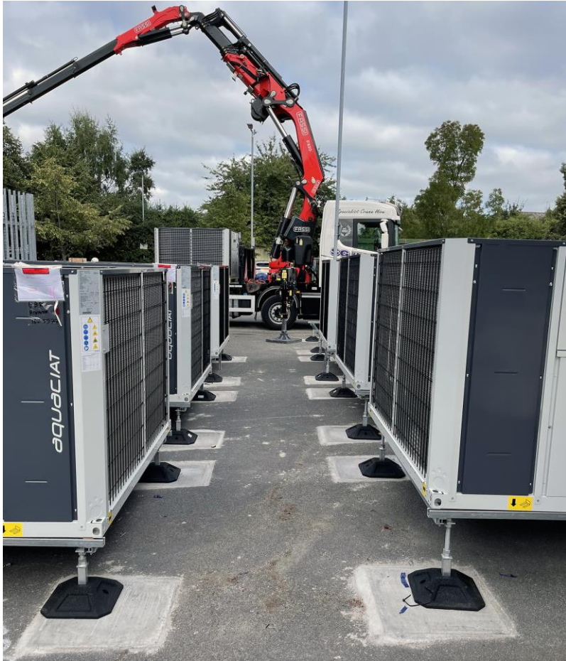
AquaCIAT units are positioned in a 'heat pump farm' at one of the larger school sites.
