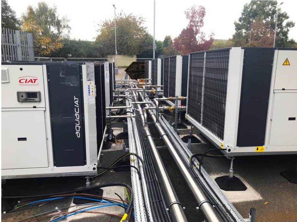
The high performance AquaCIAT heat pumps are connected up prior to lagging.
