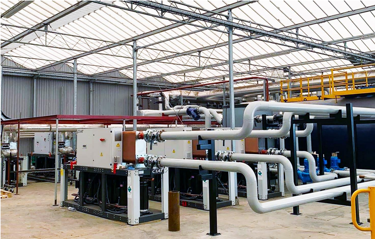
Ebtech's design is based on three DYNACIAT water-to-water units, supplied by Cool Systems Distribution Ltd.
